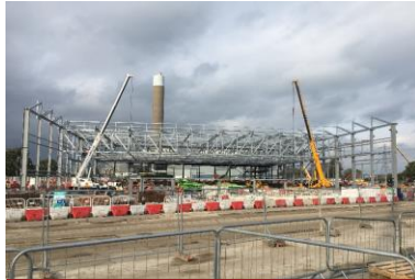
Energy from Waste - Enfield
