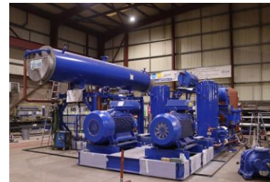
Water Source Heat Pump - Liverpool
